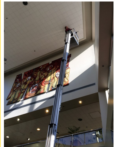
Our Electricians restored the Admin lobby lights to their original design. In short, we have light again!
