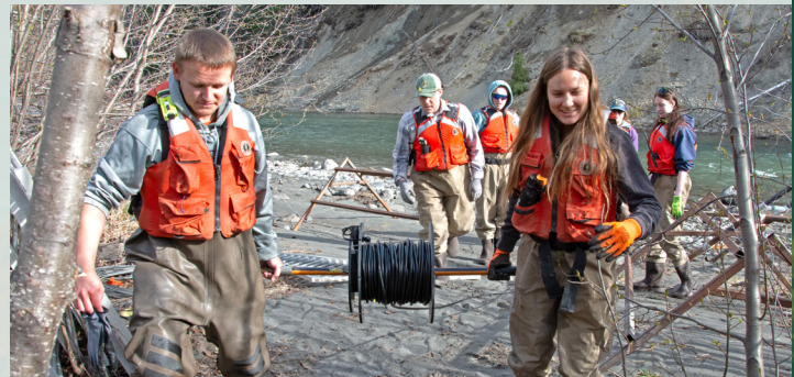
Samantha Golden, on right, helps install a sonar system on Eagle River.
